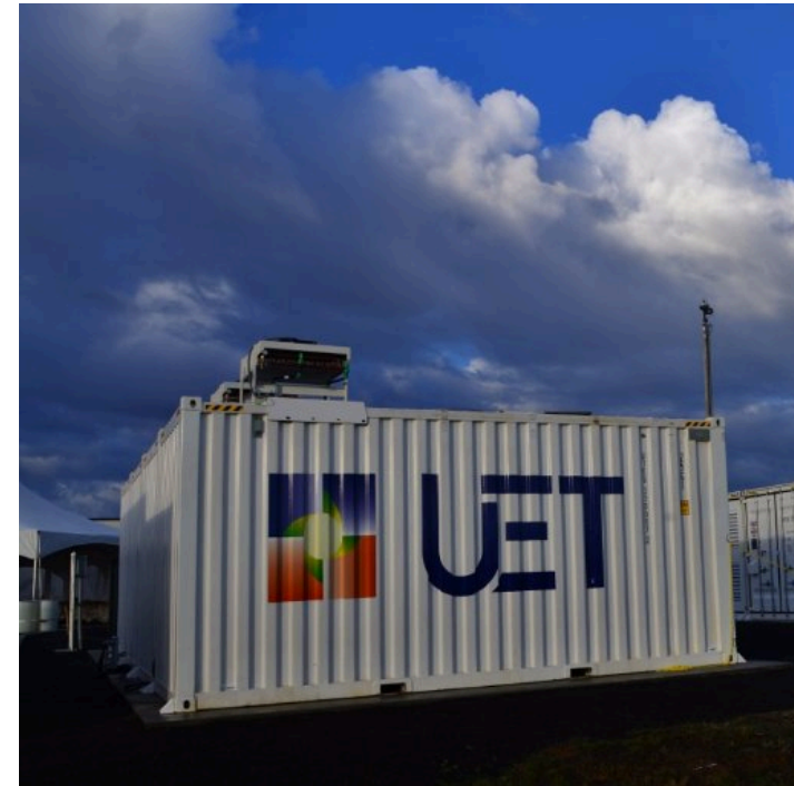
SnoPUD MESA 2 UET 2 MW/8 MWh V/V Flow
