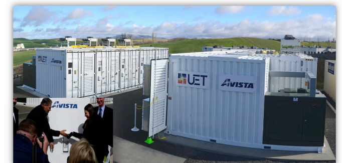
Avista Turner BESS
