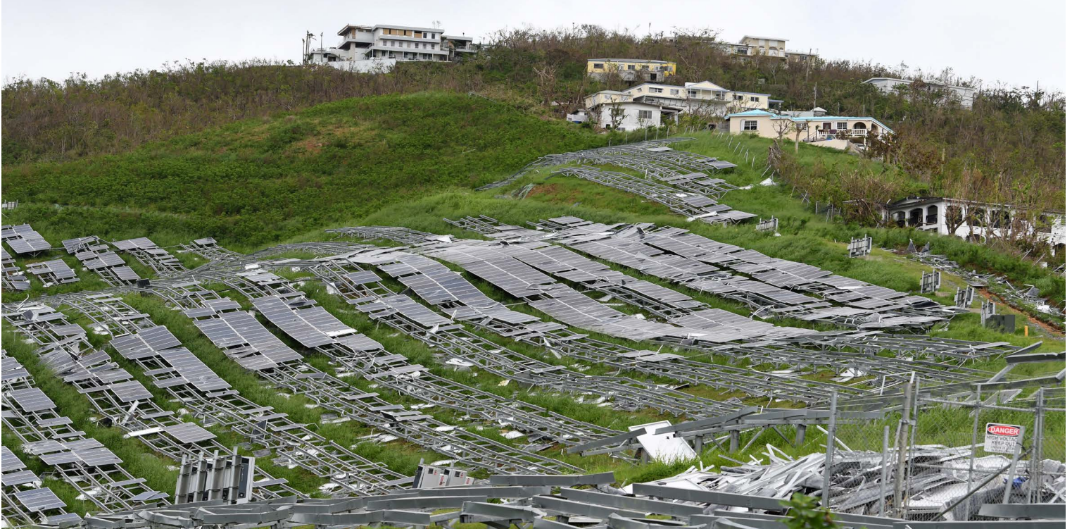
Destroyed Solar Farm on St. Thomas: 4.2 MW capacity; provided 5% of daylight power needs. Photo by Jocelyn Augustino/FEMA.
