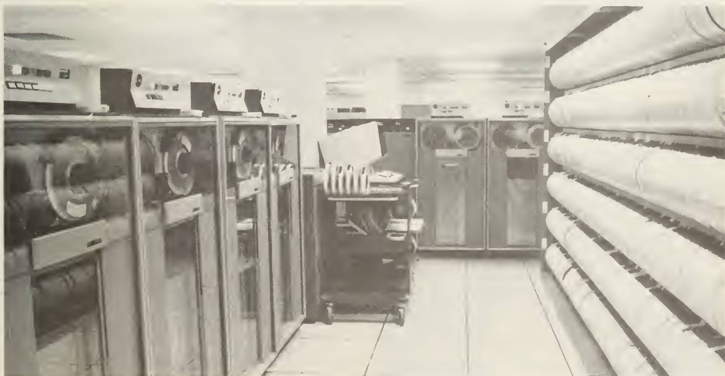
Tape Operations Area — Computer Room
